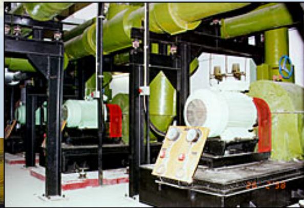
VSD for chilled water pumps
